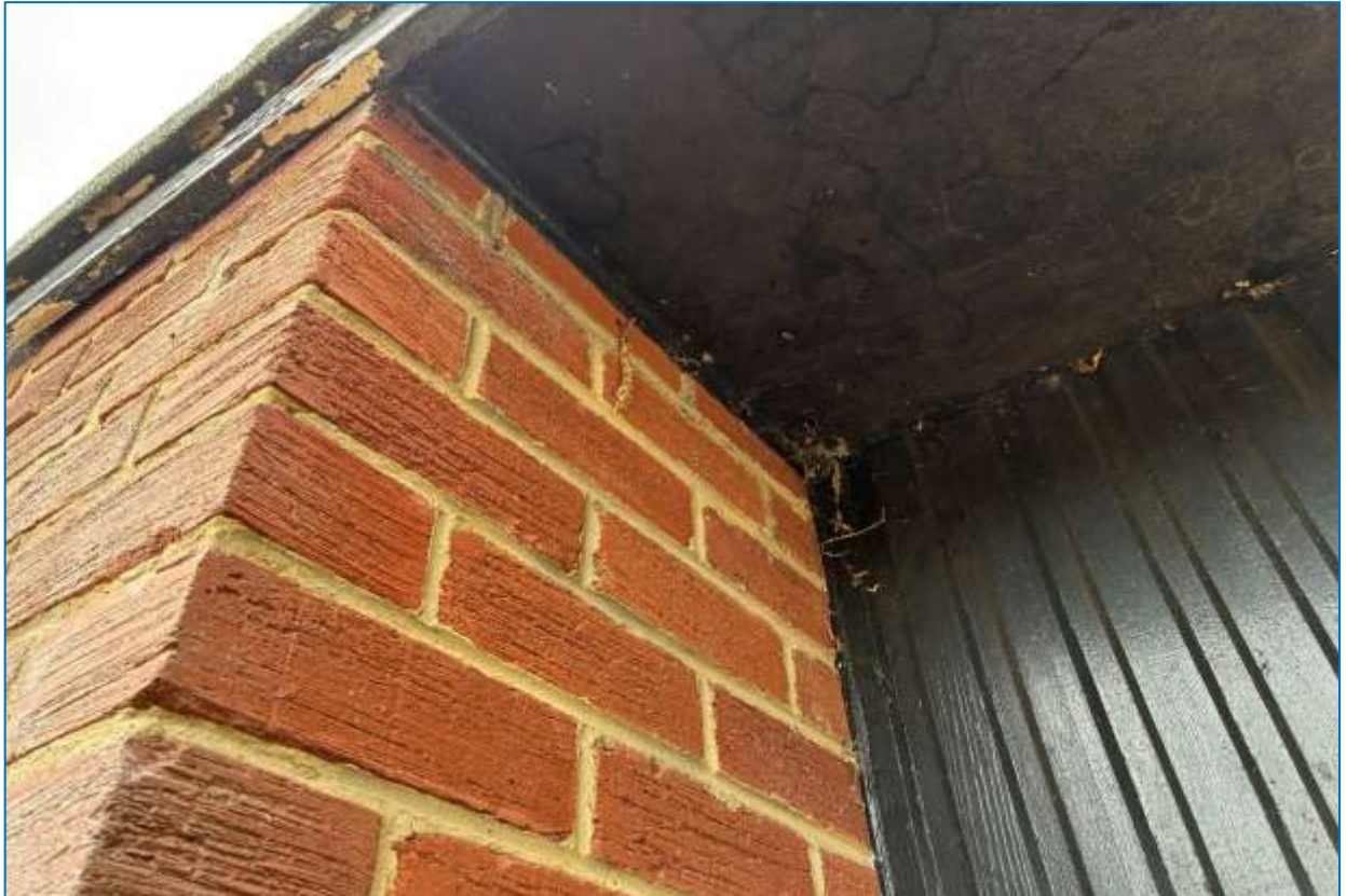
Photograph 4 – Gaps behind the fascia boards on the single storey extension.
