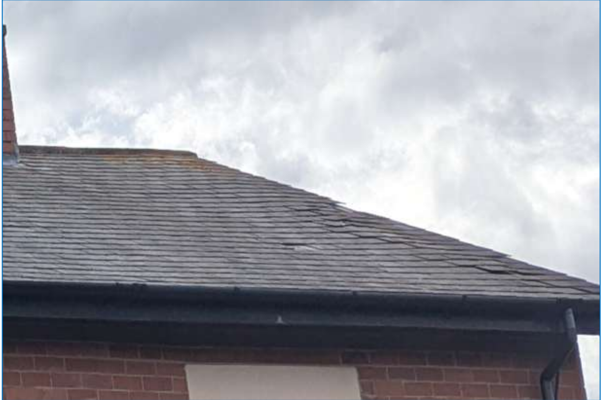
Photograph 3 – Gaps among the roof slates on the north west aspect.
