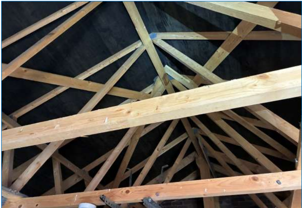
Photograph 8 – No floor present at the garage roof void.
