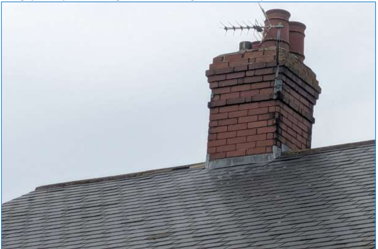
Photograph 2 – Gaps under the ridge tiles and lead flashing around the chimney.
